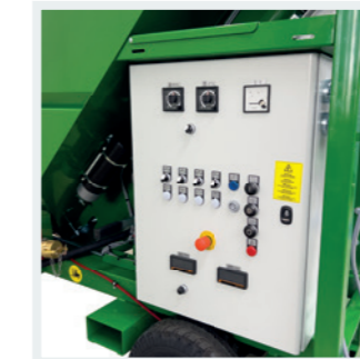
PROCESS RELIABILITY Control cabinet with timer, indicator lights and frequency converter for mixing ratios up to 10:1
